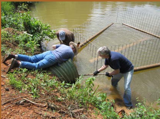
Alex Wyss (left) and Hugh Pearson excavate around the drainpipe. Judy Pearson gets a closer look at their work.
