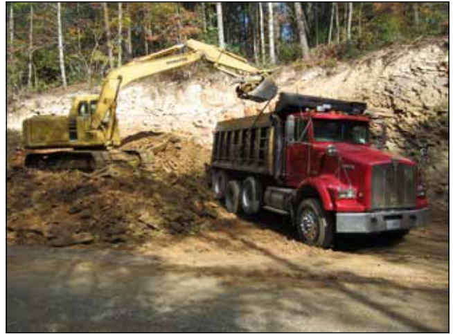
Shale fill was used from Ann Sullivan's land fronting Chilhowee Loop Road for repair of several roads.
