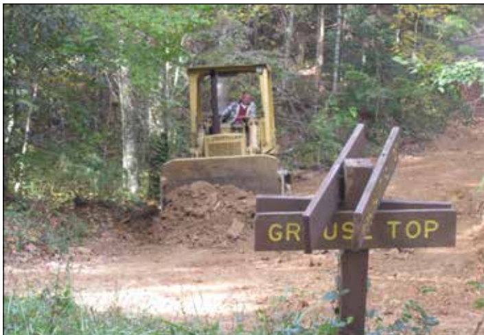
Fill being spread on Walnut Flats Road at the intersection with Grouse Top Road.
